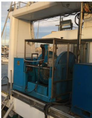
5 t SWL winch
